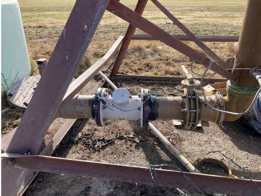
Photograph of Installed Magnetic Flow Meter at Roberti Pivot #13 Point.
